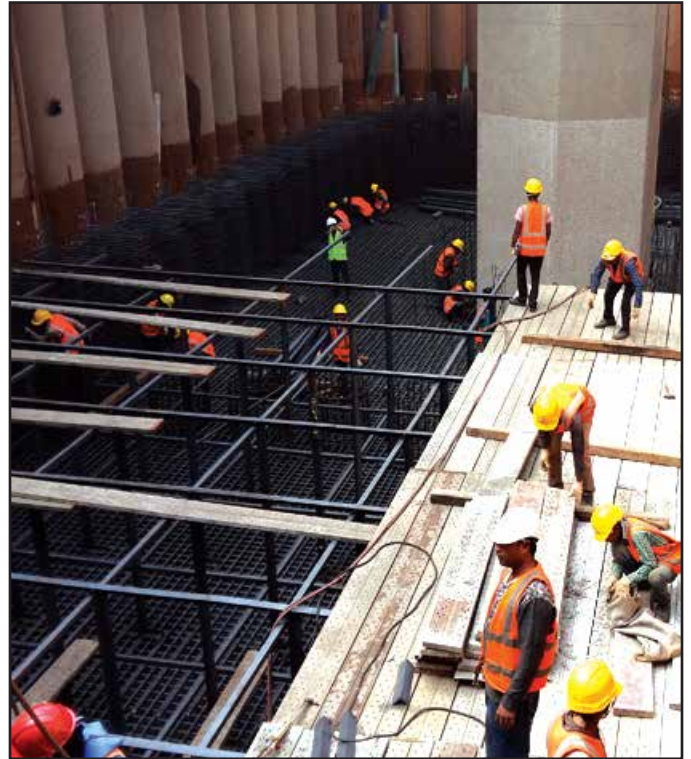
Pier- 4 Rebar Fixing for 3 rd Base Layer & Angle Frame Installation for 4 th Base Layer
