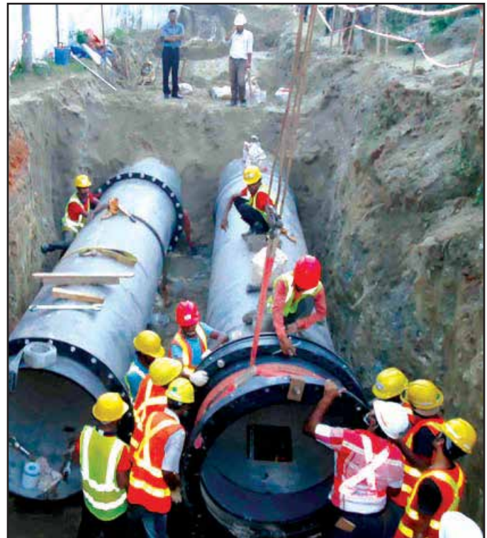
Double Line Transmission Pipeline
